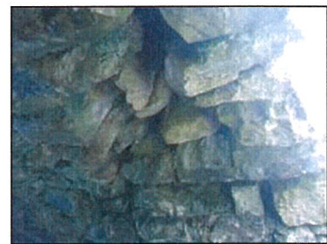
Hole in abutment and deck
