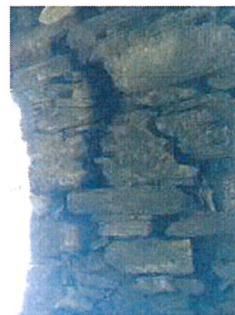
Deck and arch damage
