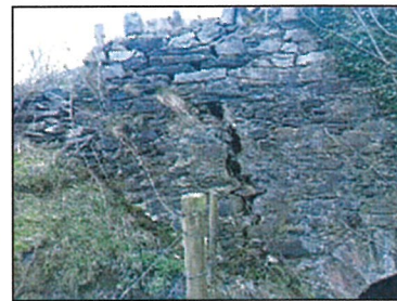
Wing wall displacement
