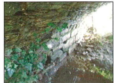
Gaps in arch abutments
