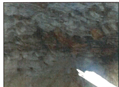
Stones dropping in soffit.
