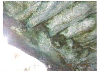
Section of arch separating
